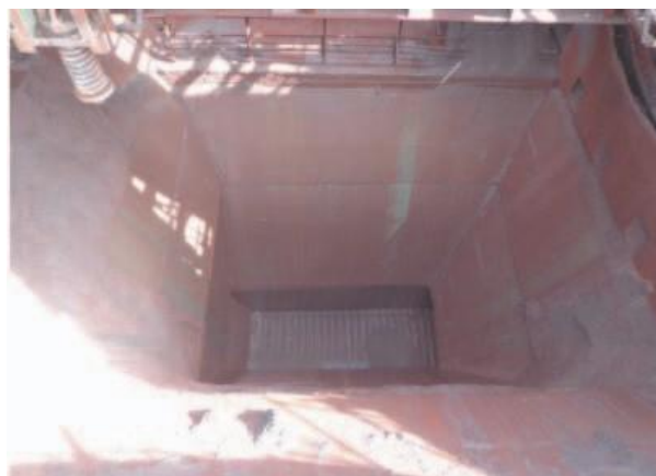
Fig. 5. FEEDER CONVEYOR CAR DUMPER
