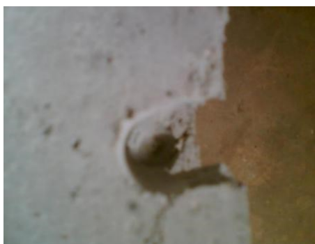
Fig. 7 Channel in the brick
