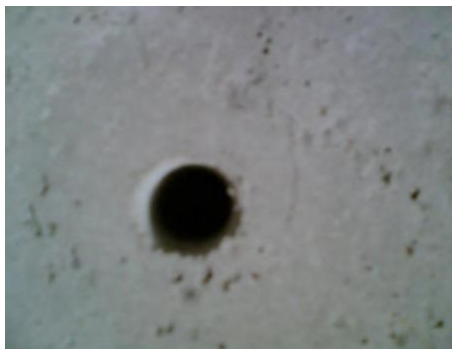
Fig. 6 Hole in the Brick
